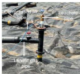
Fig. 1 Compressed air drainage well at the Taohuashan landfill
